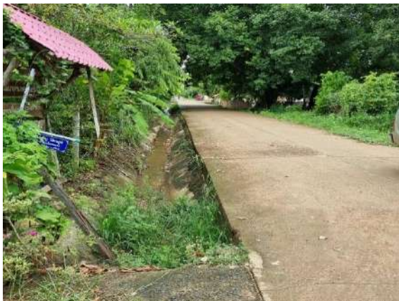
(C) A water flow road with sloped areas designed to direct water into a monkey cheek reservoir
